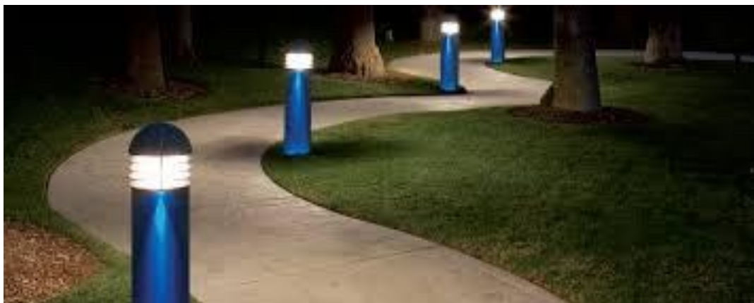
Low lighting along a pedestrian path is accomplished with pedestrian scale bollard lighting.
